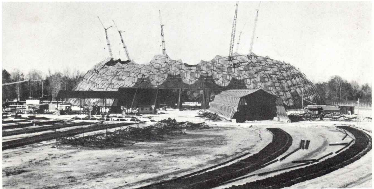
Fig. No. 78 Top: Hexagonal double grid units await installation. Units are basically same as ASM and Climatron domes substituting sheet material for inner grid and sub assembly guys. All seams are continuously welded, upper grid of sub assembly guys perform same post tensioning task as before. Four-inch tension rods make up four feet deep truss. See Fig. 102 for erection. Bottom: Frames in foreground are jigs to pre-assemble hexagonal units. Project by Synergetics Incorporated.
