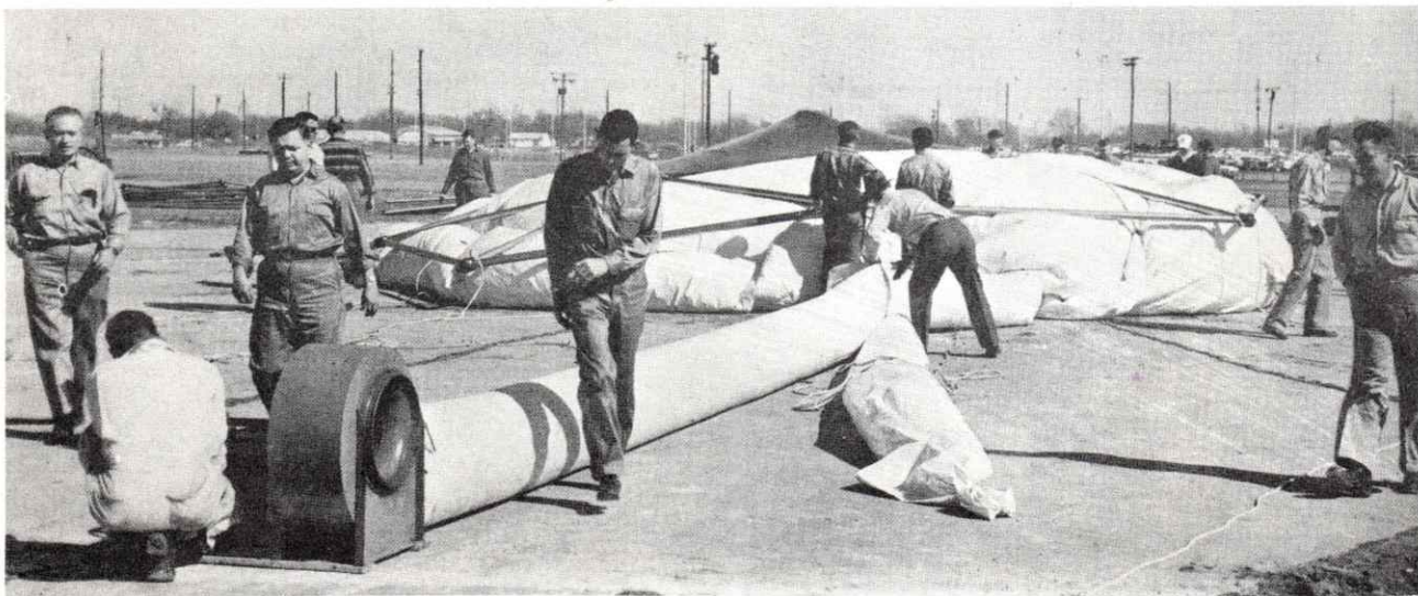
Fig. No. 97 Pneumatic balloon erection of strut dome. Zenith section bottom is anchored by guys to prevent sliding. Method proven highly successful, erectors remain on ground and near supplies. As structure raises increased perimeter enables higher numbers of simultaneous operations to be performed.
